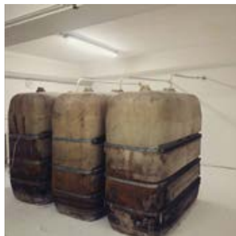
Tanks with waste oil
